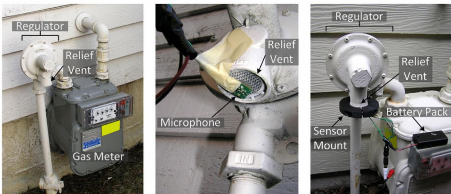
Fig. 1. (left) A typical US gas meter and pressure regulator. (middle) The location of our microphone-based sensor on the pressure regulator relief vent. (right) The GasSense prototype and sensor mount attached to the relief vent.
